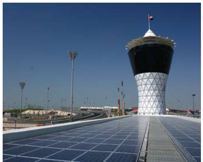
Shams Tower Solar Roof, Yas Marina Circuit, Abu Dhabi, installed by Enviromena
