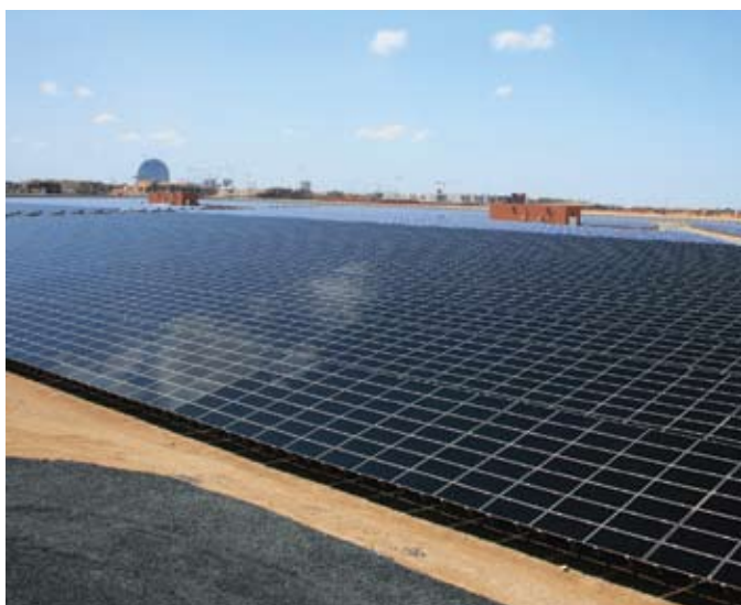
Masdar 10MW Solar Power Plant, Abu Dhabi, constructed by Enviromena
